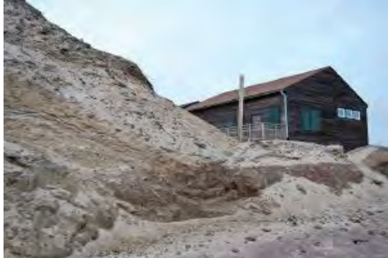
Wear and storm undermining has resulted in boardwalk repair in 1989, 1991, 1992, 1993, 1996 and in 2000. Photo by Hannah Vahl
